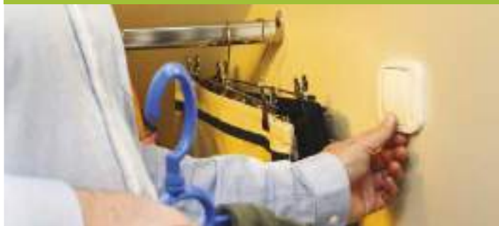
Creation of a new back-and-forth with a wireless and battery-less wall switch
